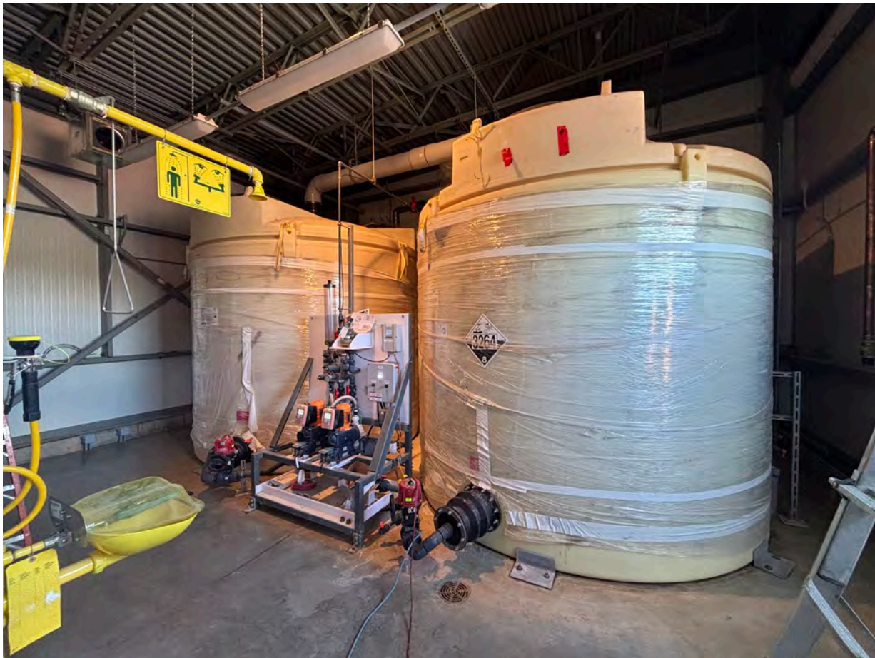
Figure 2: New Alum Tanks and pump skid
